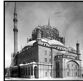
c) After casting the domes and semi-domes and before casting the central dome.
